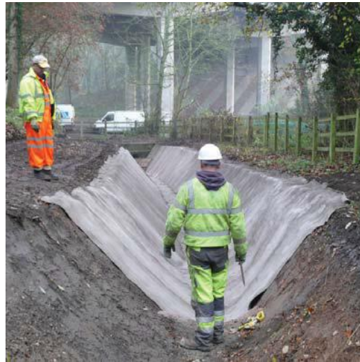
M4 interceptor drain lining: M4, Wiltshire, UK
